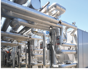
Viking technicians devised this elaborate piping for the absorption chiller, which produces plant cooling for the company's tri-generation system.
