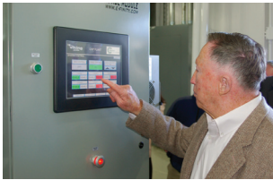
Viking president and co-founder Bill Healey demonstrates the custom touch-screen control panel, which flows electricity and hot water throughout the building.
